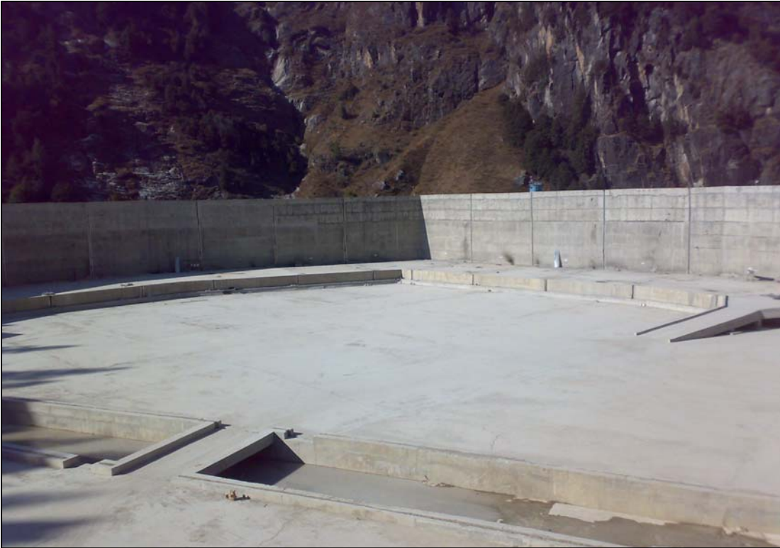
D-15: A view of constructed Intermediate Reservoir
